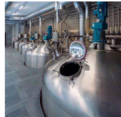
Mixing tanks - 3m 3 , 3m 3 , 6m 3 , 10 m 3 , 32 m 3
